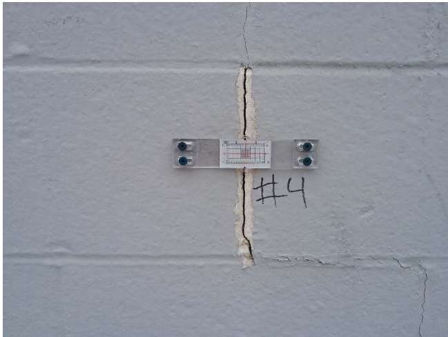
Photo 7: Crack gauge 4 position on a vertical crack on the north exterior wall.
