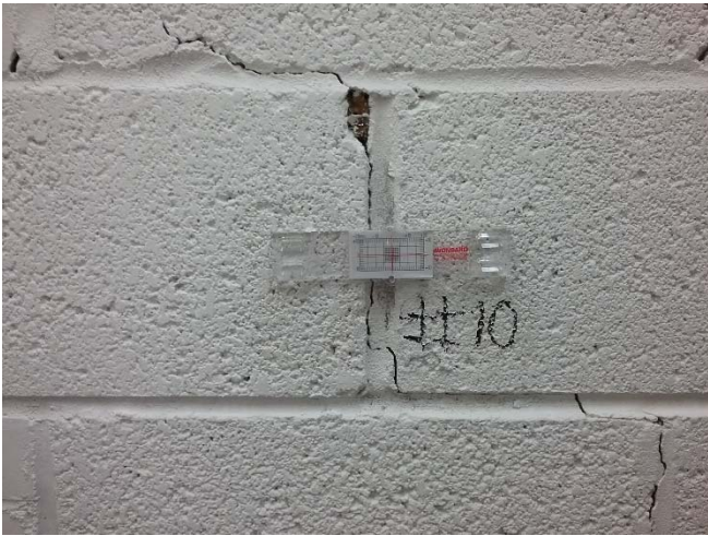
Photo 19: Crack gauge 10 position on a diagonal crack in an interior storage room.
