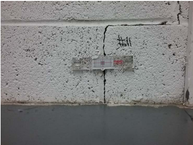
Photo 21: Crack gauge 11 position on a low diagonal crack inside the electrical room.
