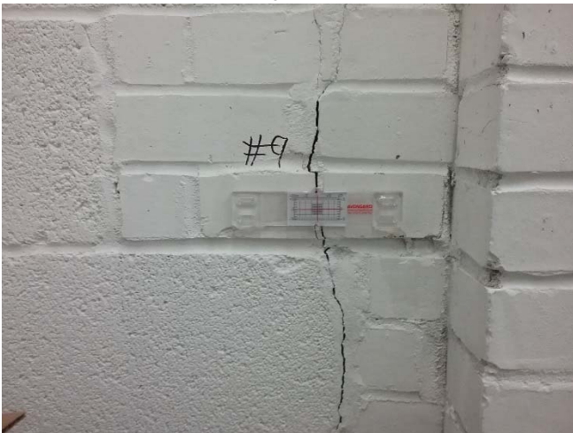
Photo 17: Crack gauge 9 position on a vertical crack in an interior storage room.
