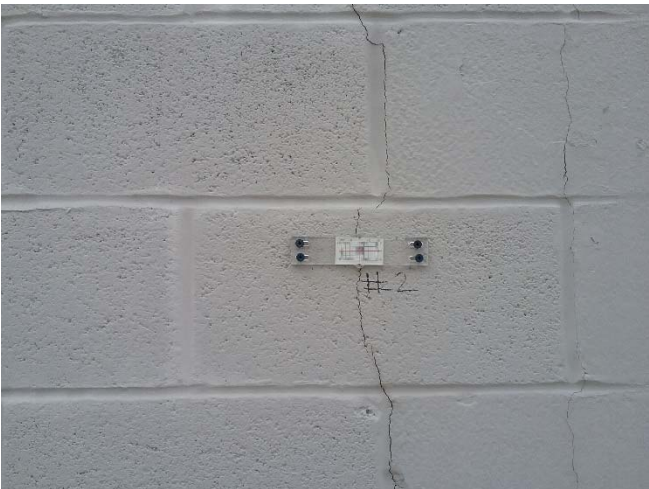
Photo 3: Crack gauge 2 position on a vertical crack on the north exterior wall.
