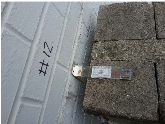
Photo 23: Crack gauge 12 positioned between the wall and the exterior west staircase.
