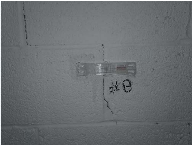
Photo 15: Crack gauge 8 position on a diagonal crack in an interior storage room.
