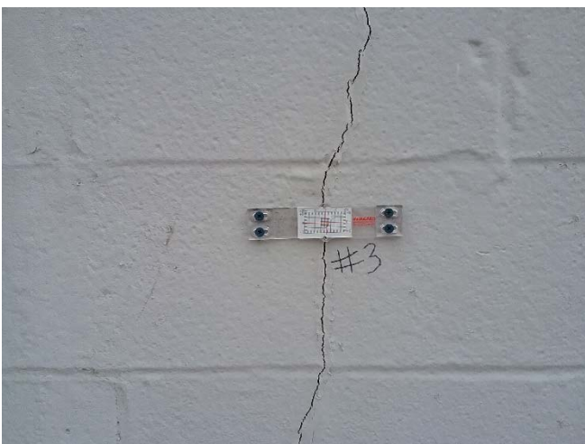
Photo 5: Crack gauge 3 position on a vertical crack on the north exterior wall.
