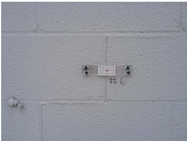
Photo 11: Crack gauge 6 position on a diagonal crack on the north exterior wall.
