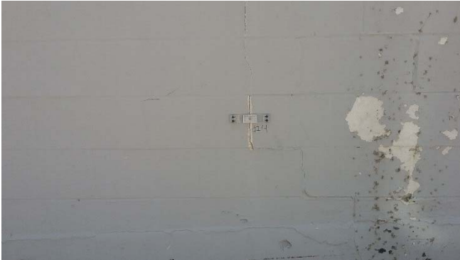
Photo 7: Crack gauge 4 position on a vertical crack on the north exterior wall.
