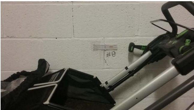
Photo 15: Crack gauge 8 position on a diagonal crack in an interior storage room.
