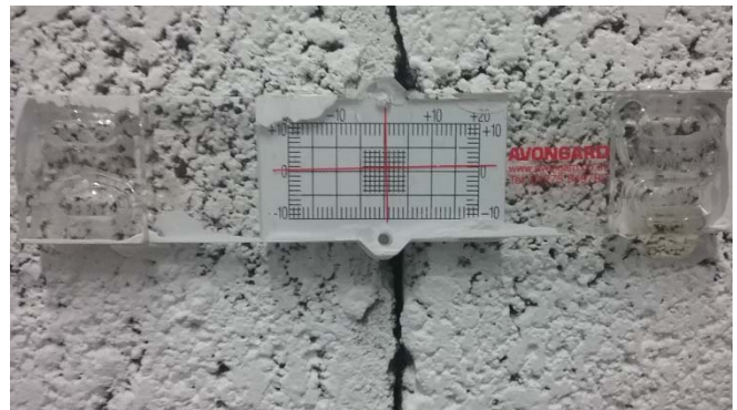
Photo 22: Close up view of crack gauge 11.
