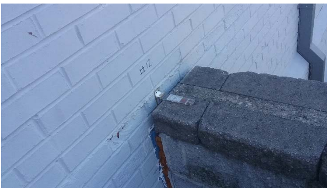
Photo 23: Crack gauge 12 positioned between the wall and the exterior west staircase.
