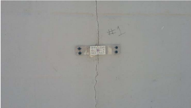
Photo 1: Crack gauge 1 position on a vertical crack on the north exterior wall.
