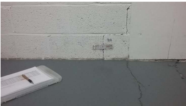
Photo 21: Crack gauge 11 position on a low diagonal crack inside the electrical room.
