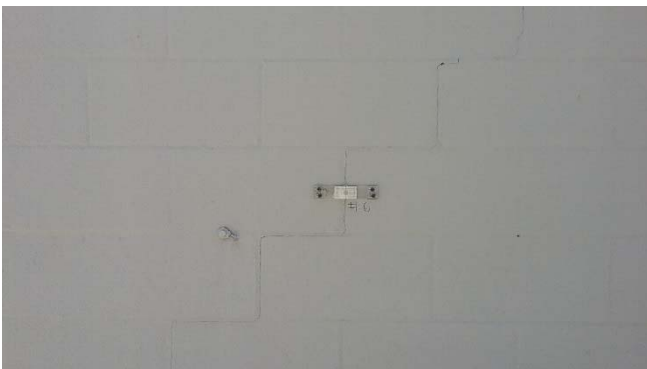
Photo 11: Crack gauge 6 position on a diagonal crack on the north exterior wall.
