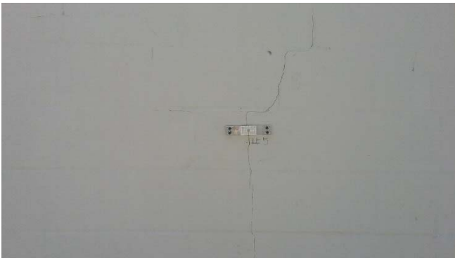
Photo 9: Crack gauge 5 position on a vertical crack on the north exterior wall.
