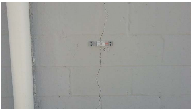
Photo 5: Crack gauge 3 position on a vertical crack on the north exterior wall.
