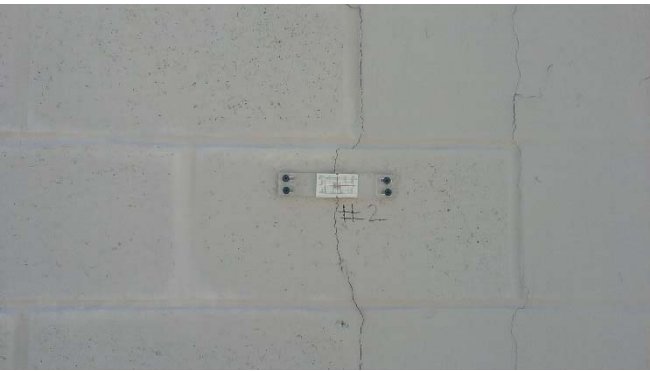
Photo 3: Crack gauge 2 position on a vertical crack on the north exterior wall.
