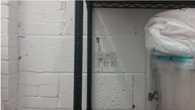
Photo 19: Crack gauge 10 position on a diagonal crack in an interior storage room.
