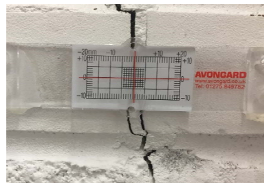
Photo 18: Close up view of crack gauge 9.
