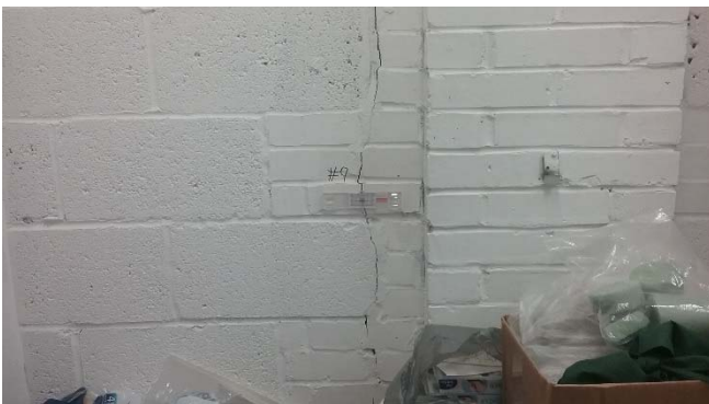
Photo 17: Crack gauge 9 position on a vertical crack in an interior storage room.
