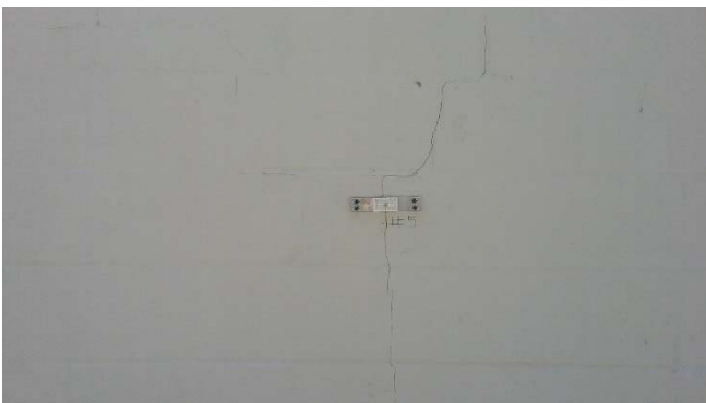
Photo 9: Crack gauge 5 position on a vertical crack on the north exterior wall.
