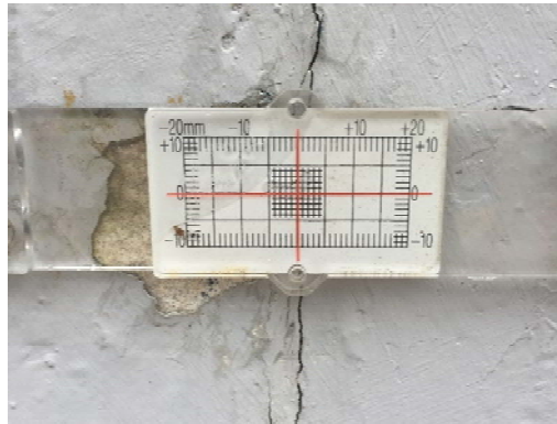
Photo 2: Close up view of crack gauge 1.
