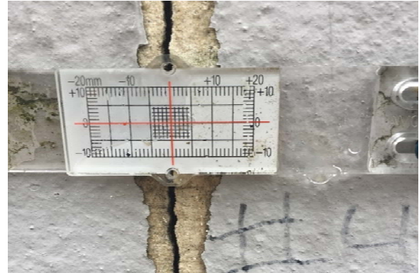
Photo 8: Close up view of crack gauge 4.
