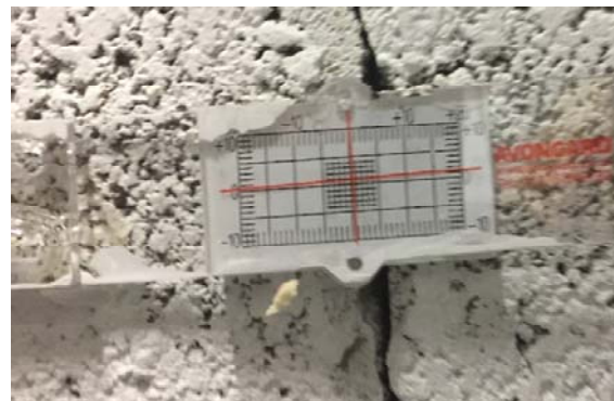
Photo 22: Close up view of crack gauge 11.
