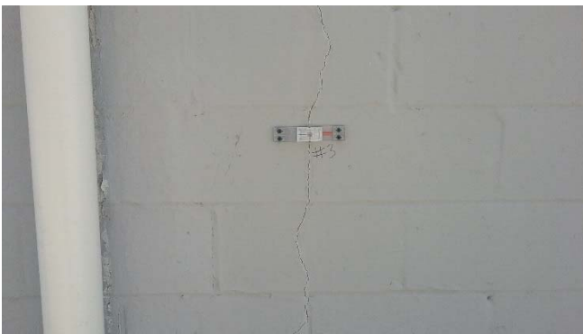
Photo 5: Crack gauge 3 position on a vertical crack on the north exterior wall.
