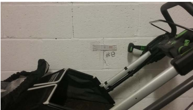
Photo 15: Crack gauge 8 position on a diagonal crack in an interior storage room.
