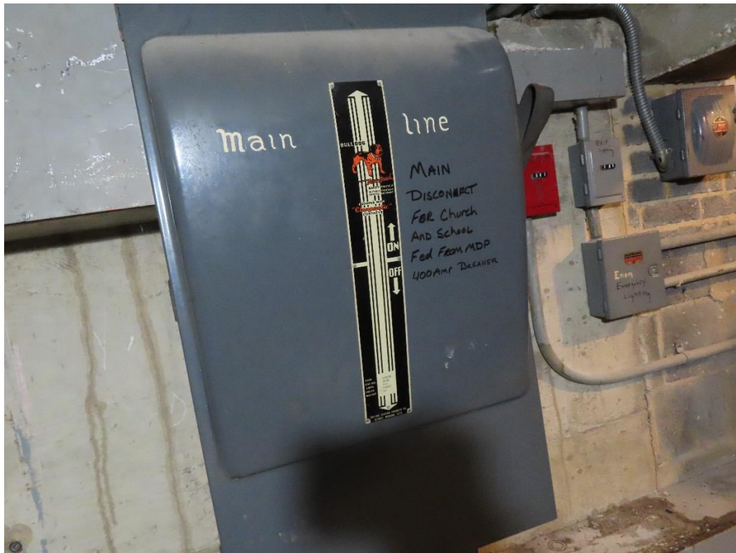
Photograph 37: Bulldog disconnect switch
