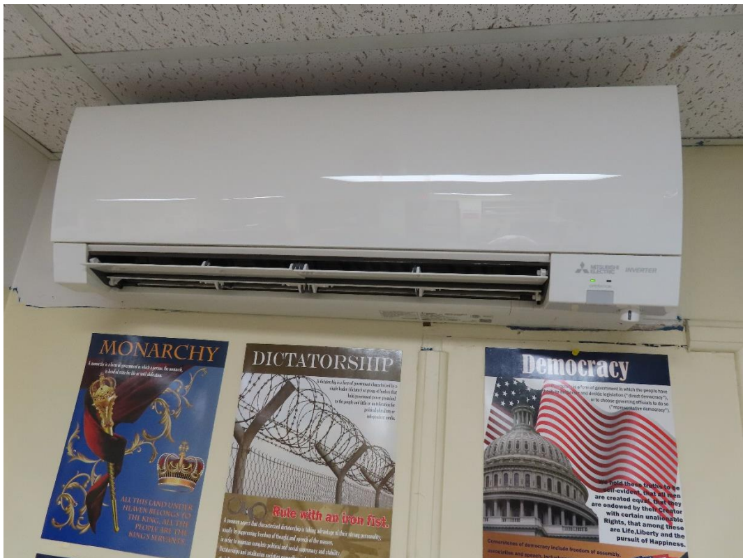
Photograph 32: Mini-split interior air fan coil unit
