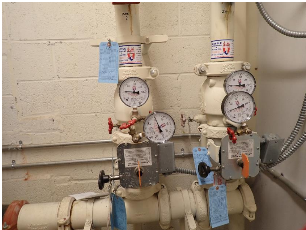
Photograph 42: Sprinkler system risers.
