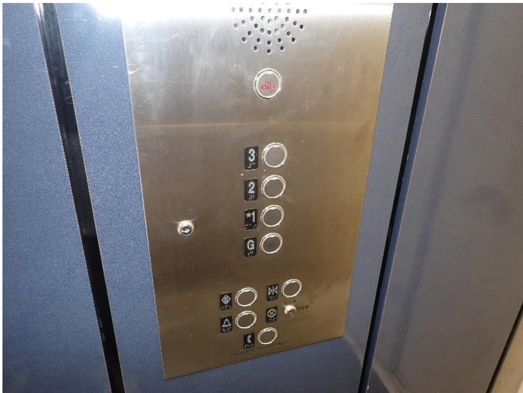
Photograph 46: Elevator car control panel.
