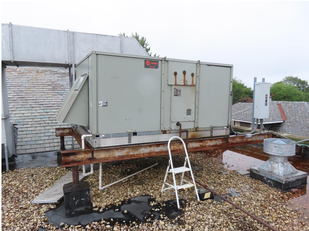
Photograph 22: 12.5 ton rooftop package unit.
