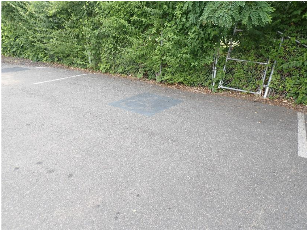
Photograph 9: Typical site asphalt - note non-compliant ADA parking stall
