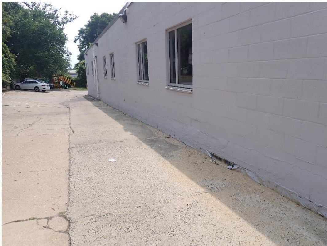
Photograph 8: Cracked concrete paving.
