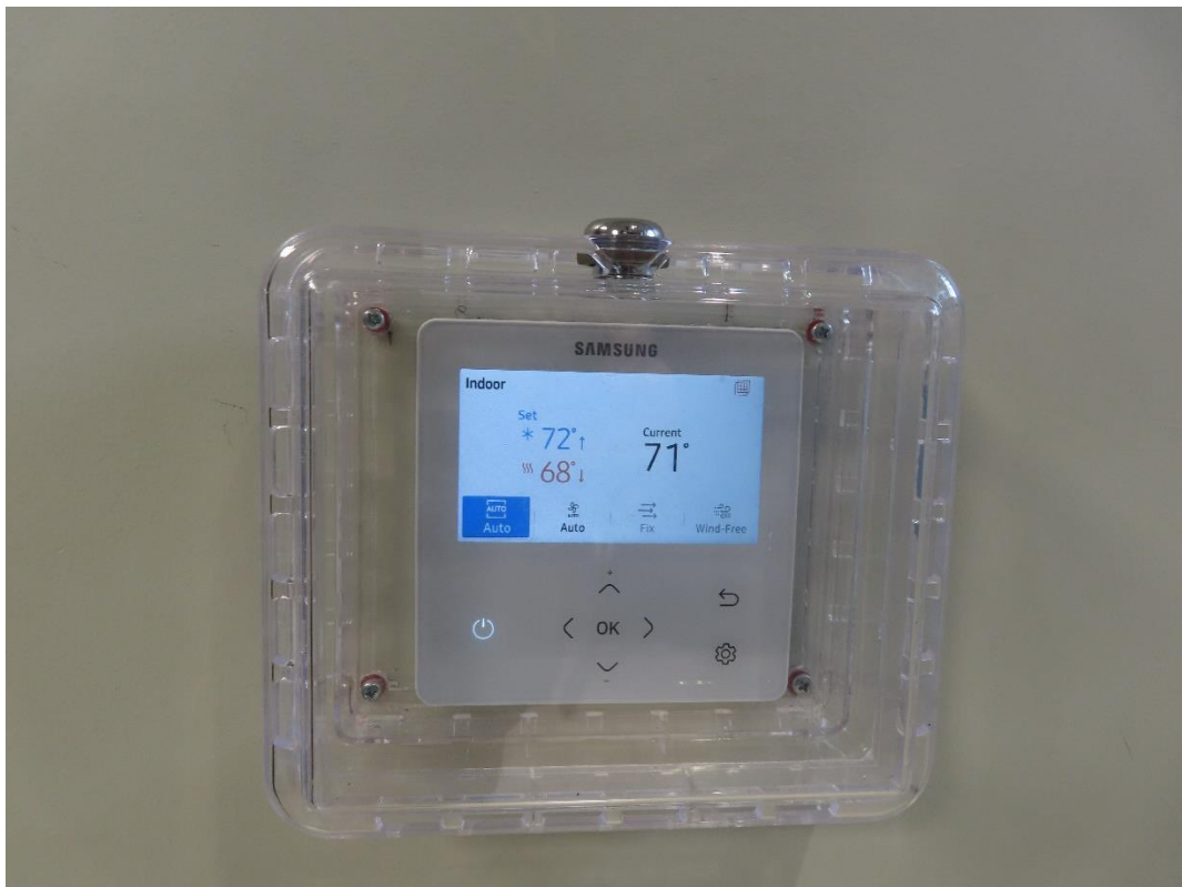
Photograph 34: VRF control thermostat.
