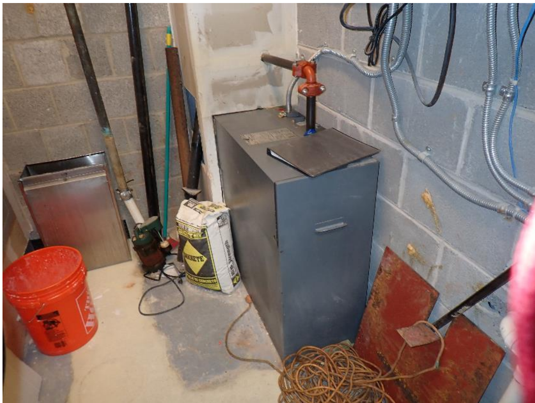
Photograph 48: Elevator hydraulic pump unit.
