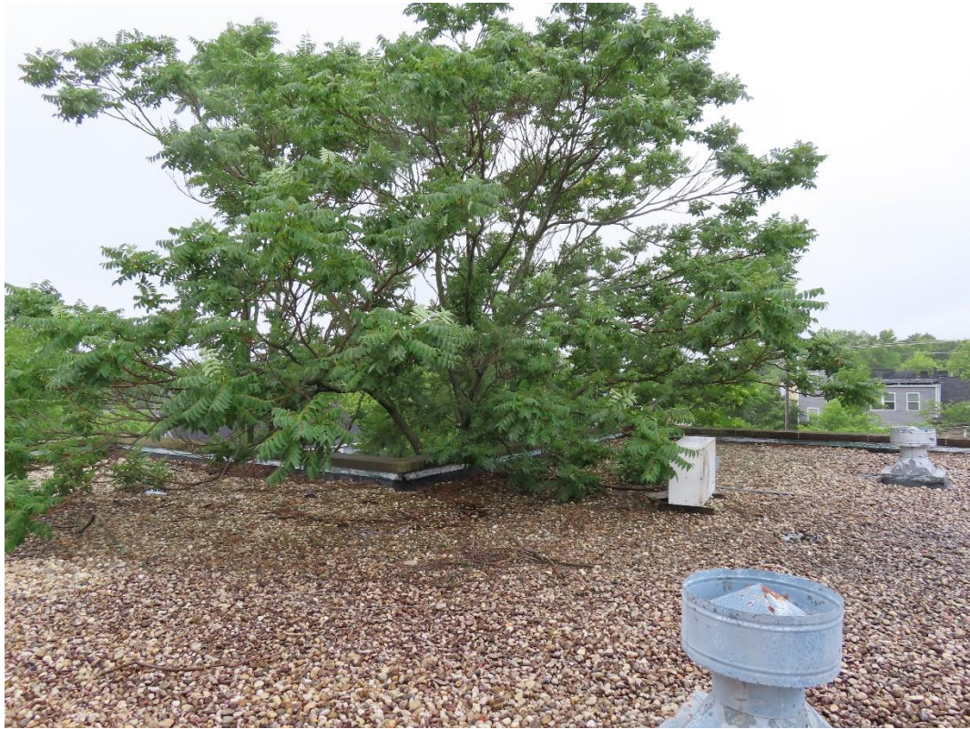
Photograph 7: Encroaching trees on roof.
