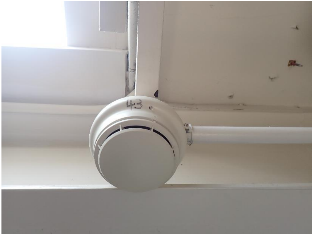
Photograph 45: Typical smoke alarm.
