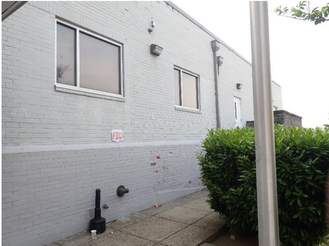
Photograph 20: Typical exterior wall and window systems. Note localized spalled bricks
