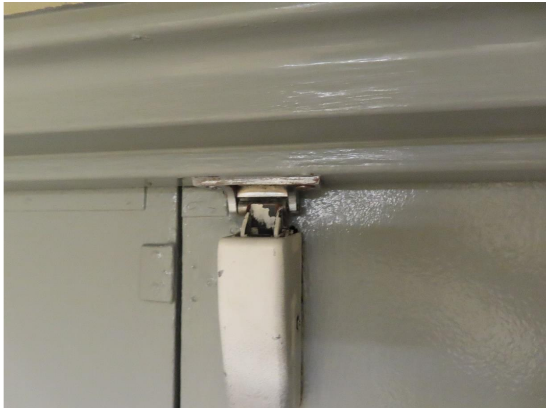
Photograph 48: Inoperable emergency egress hardware.
