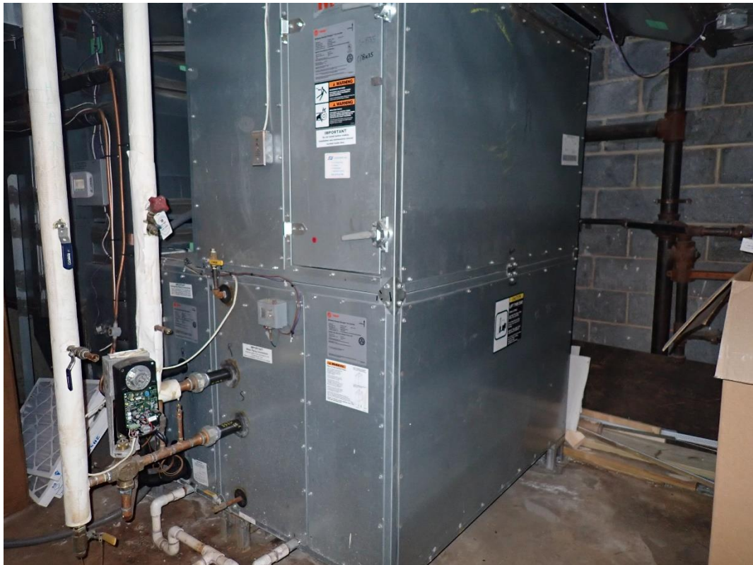
Photograph 24: Trane air-handling unit.
