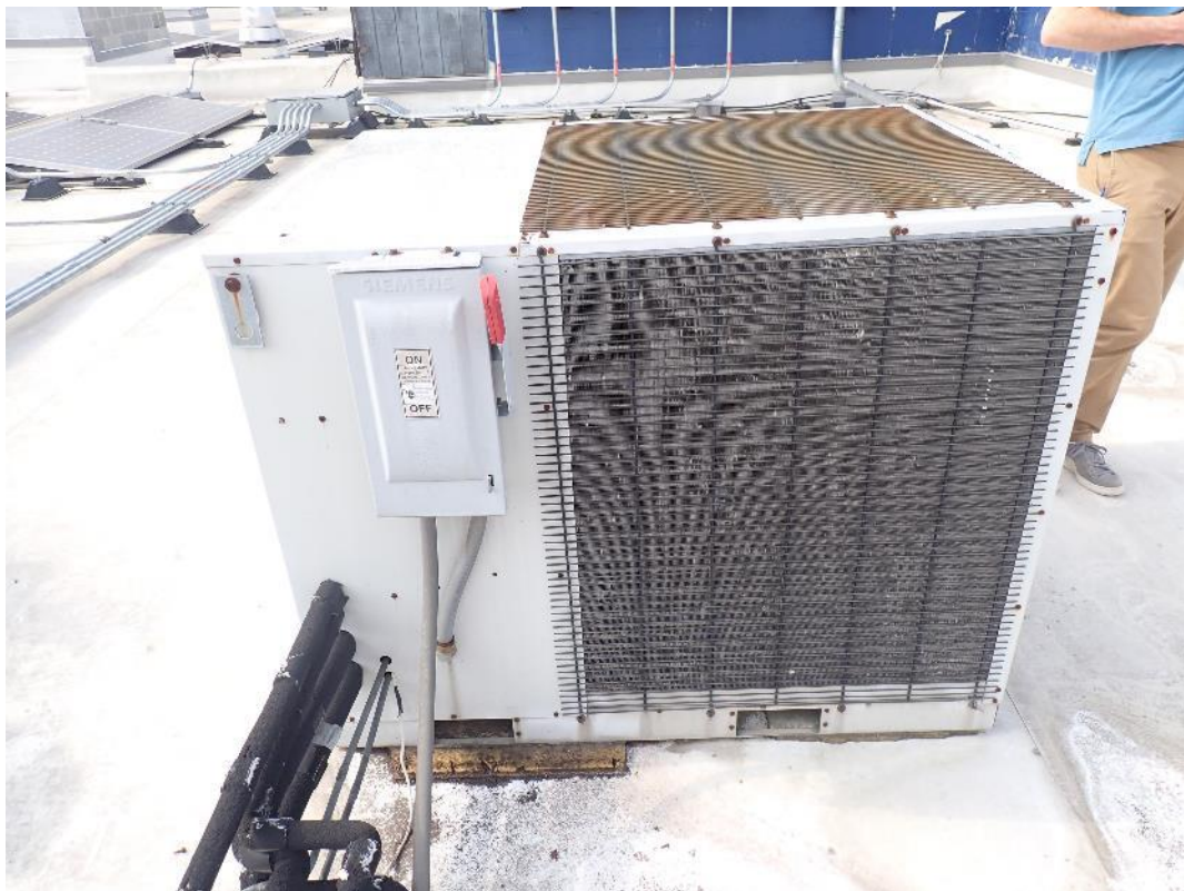
Photograph 30: Exterior condensing unit which serves one of two split systems.
