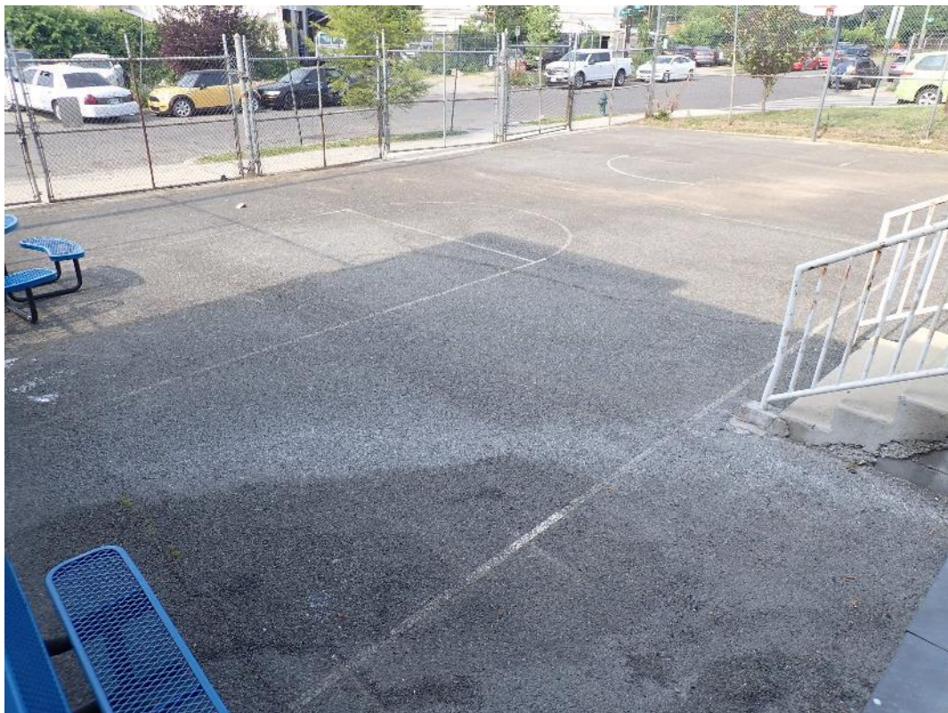
Photograph 6: Asphalt at rear basketball court.
