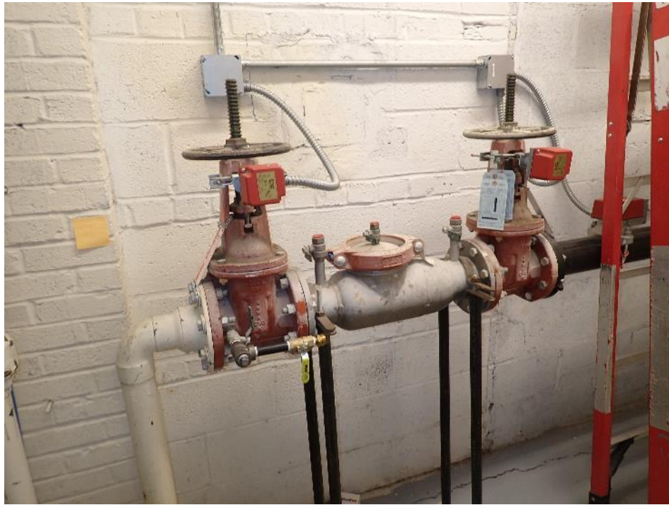
Photograph 41: Incoming sprinkler pipework.
