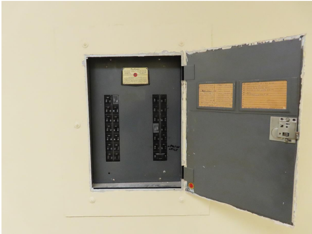
Photograph 35: Bulldog Pushmatic Breaker panel.
