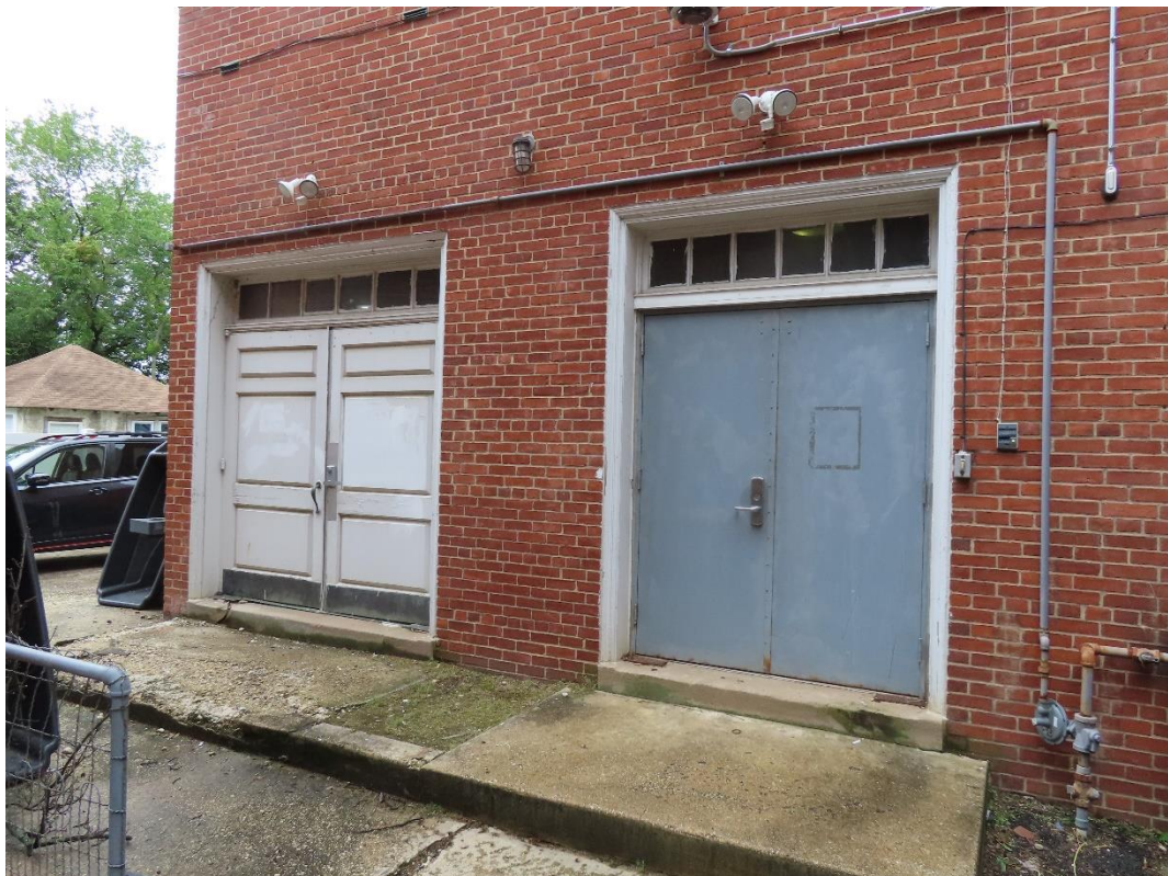
Photograph 6: Deteriorated concrete at step
