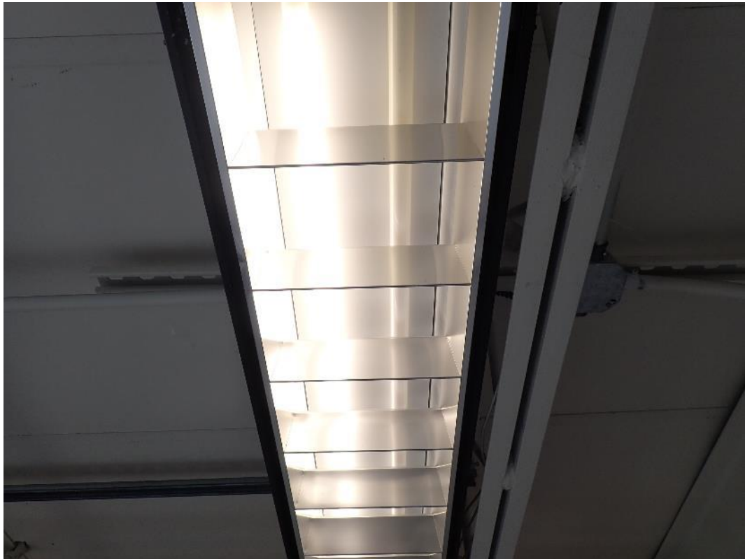
Photograph 39: Older fluorescent lighting.
