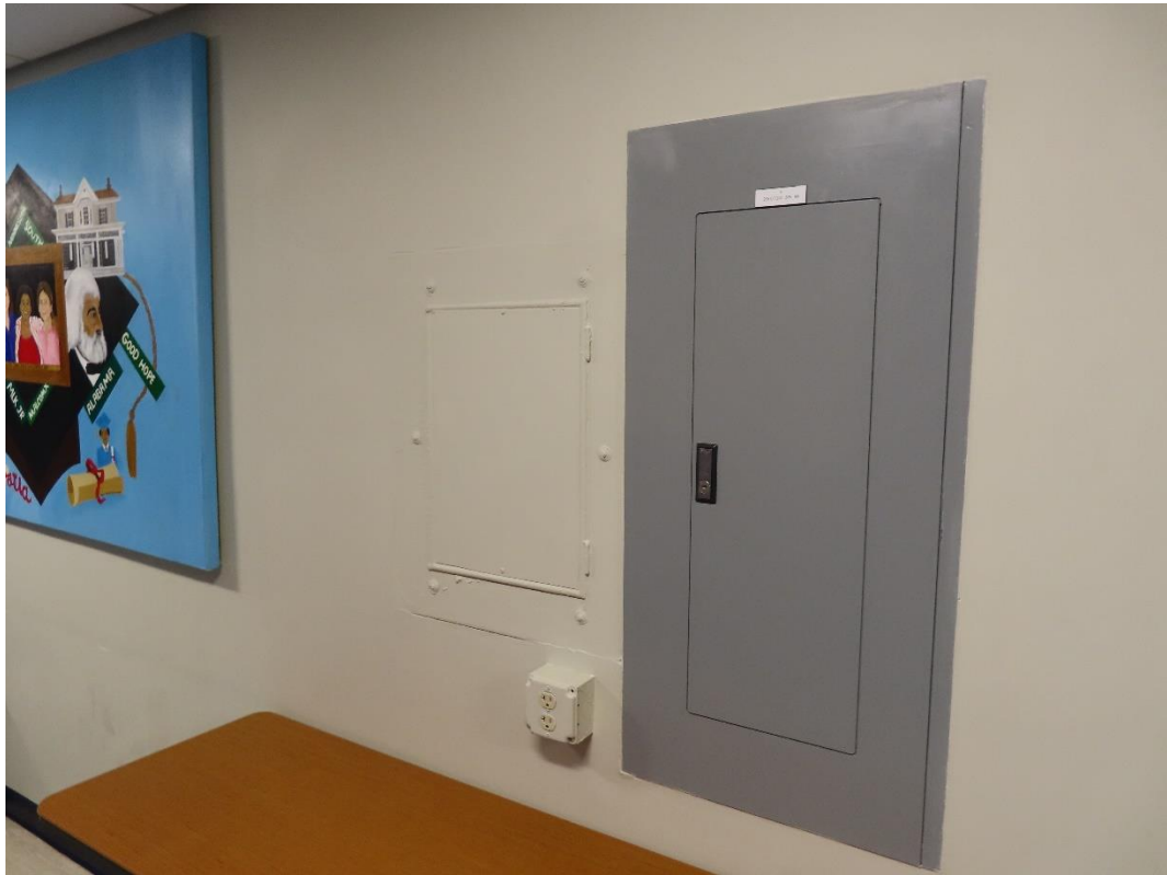
Photograph 42: New breaker panel in lobby.
