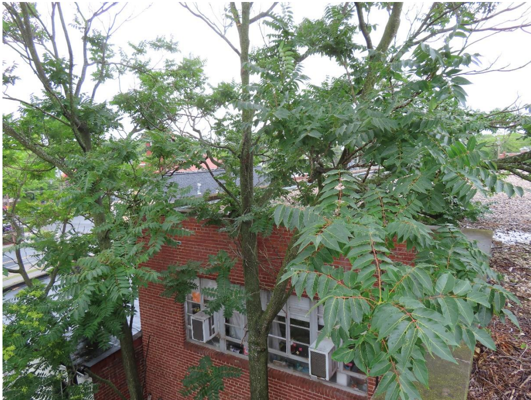
Photograph 8: Trees encroaching on roof.
