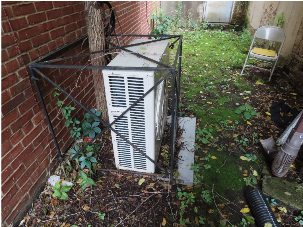
Photograph 33: Mini-split external condenser unit.
