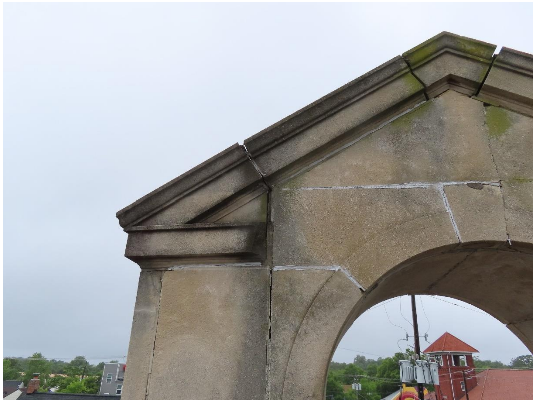
Photograph 15: Open mortar joints and previous joint repair to bell tower.
