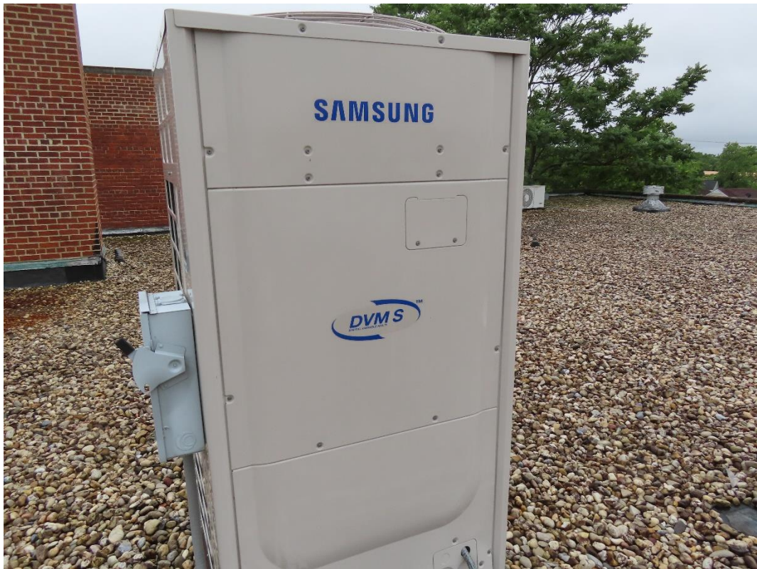
Photograph 31: 6 Ton VRF split heat pump unit.
