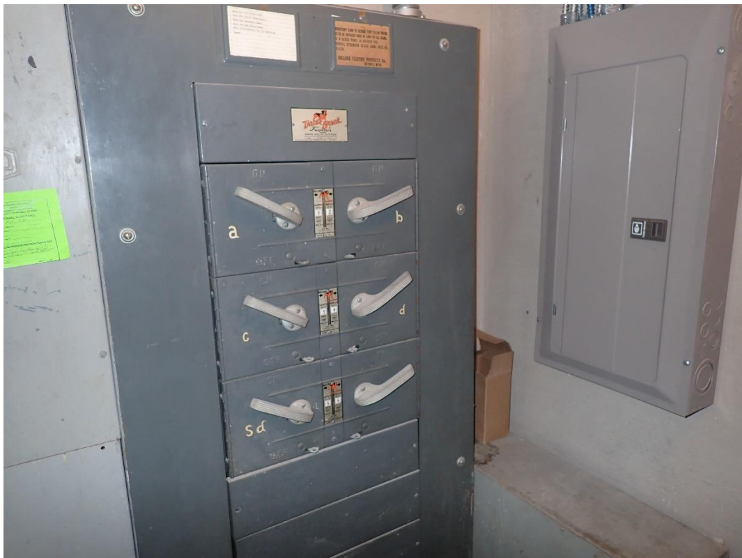
Photograph 36: Bulldog 400 amp main disconnect.
