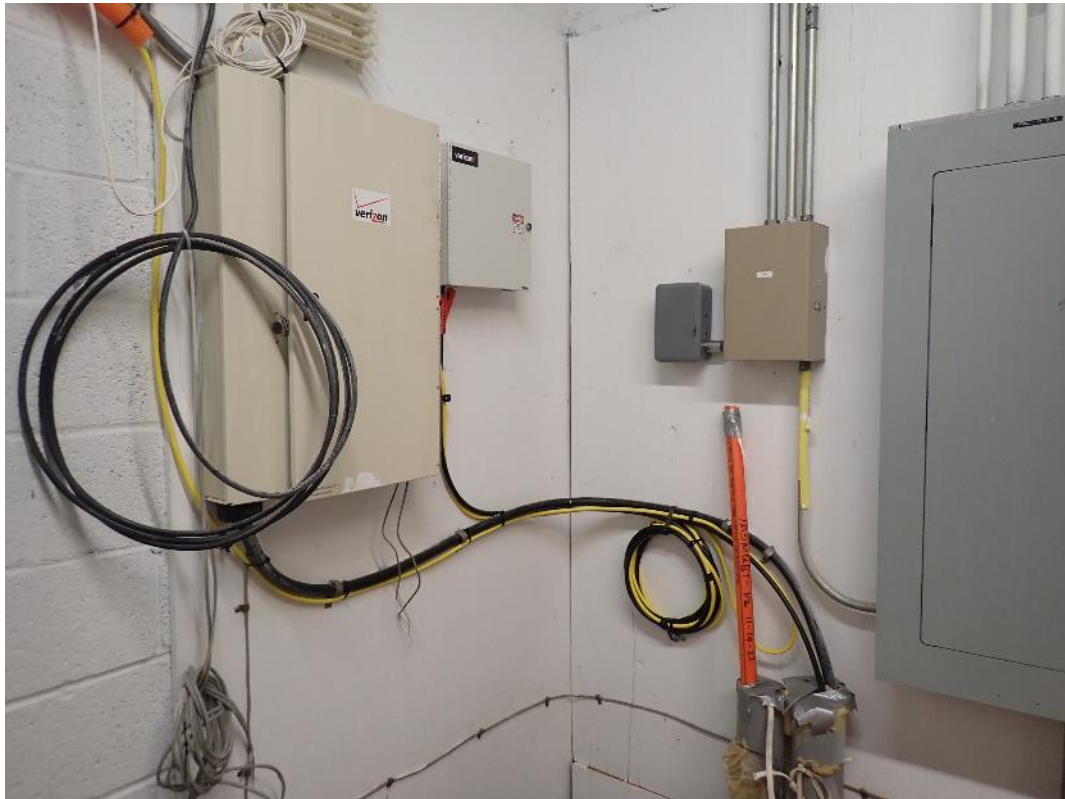
Photograph 37: Telecoms and data systems.
