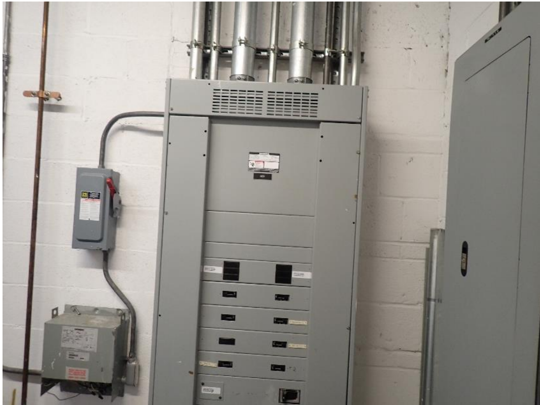
Photograph 35: Main distribution panel.
