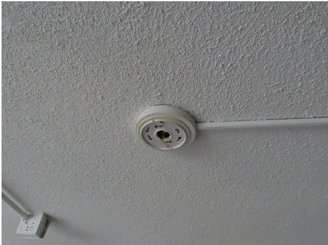
Photograph 50: Missing detector head in classroom.
