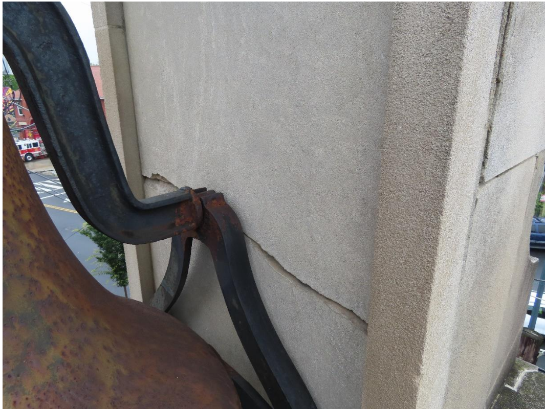
Photograph 17: Cracked stone panel and panel movement.
