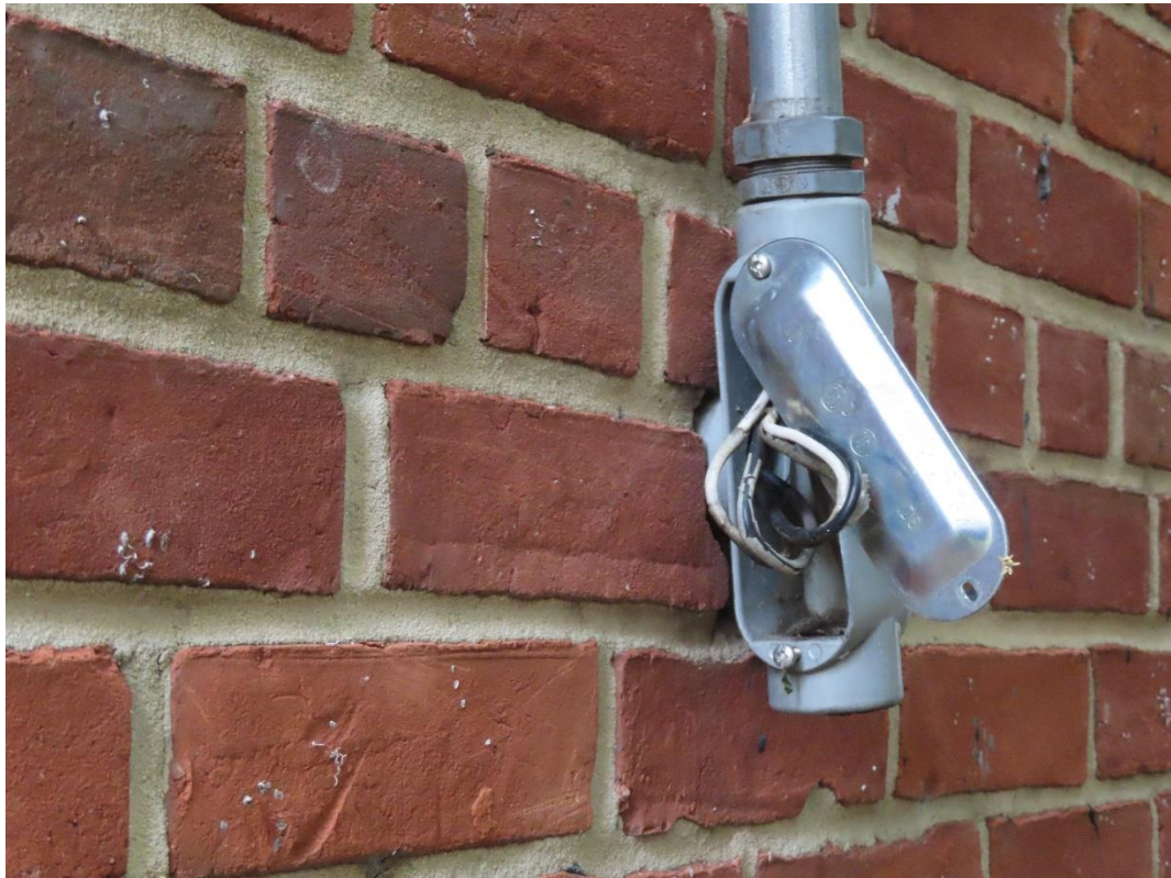
Photograph 39: Open electrical junction box.
