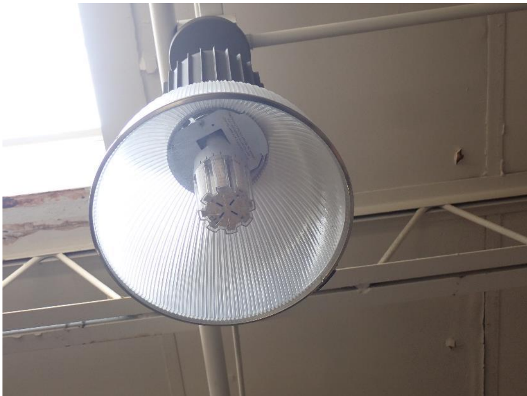
Photograph 38: Light fitting retrofitted with LED bulb.
