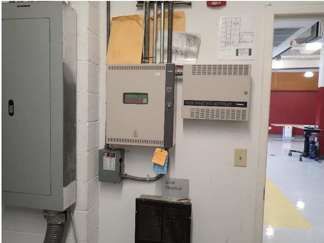
Photograph 43: Fire alarm control panel.
