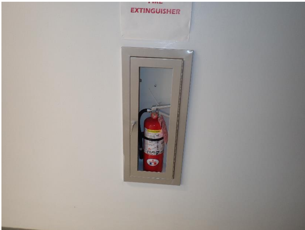
Photograph 44: Handheld fire extinguisher.
