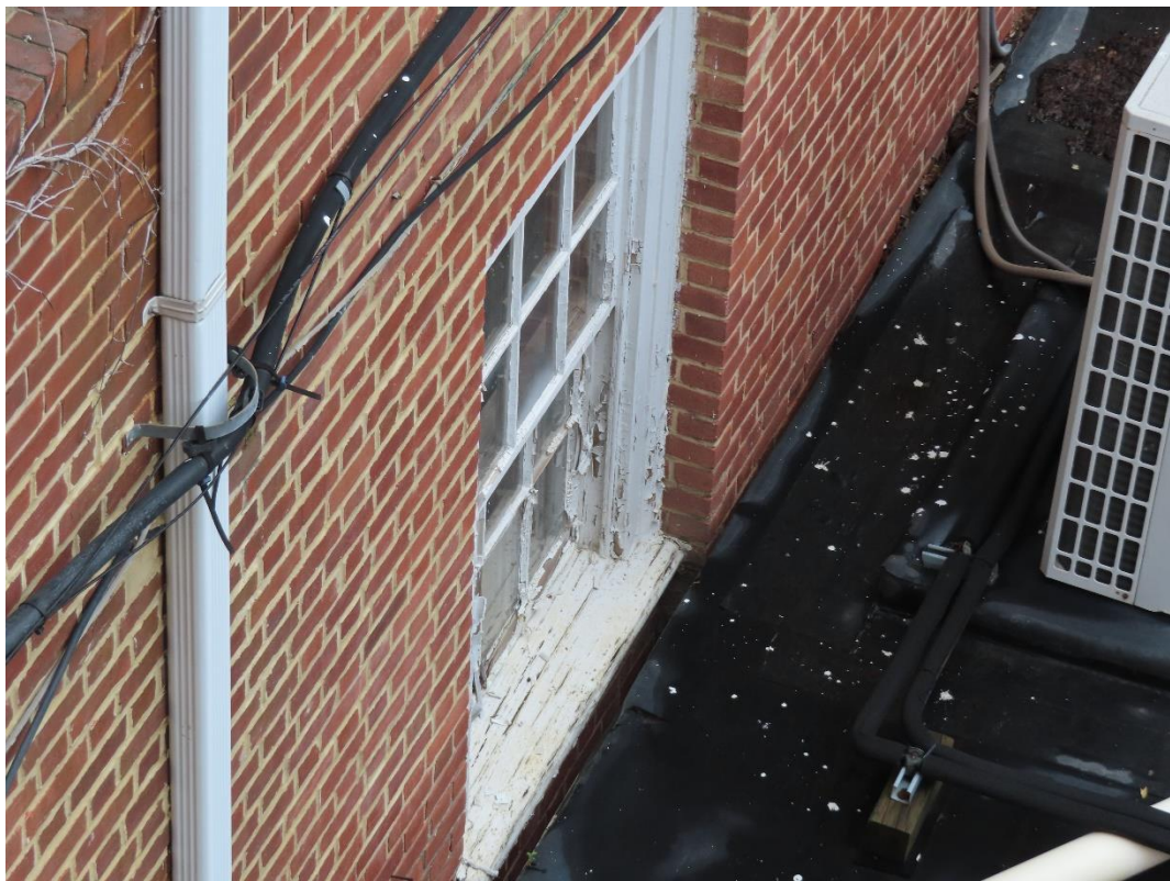
Photograph 18: Flaking paint to wood windows.
