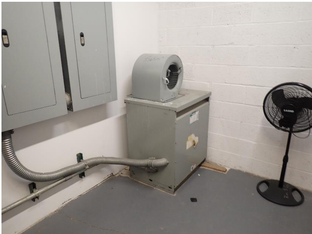
Photograph 36: Panelboards and step-down transformer.
