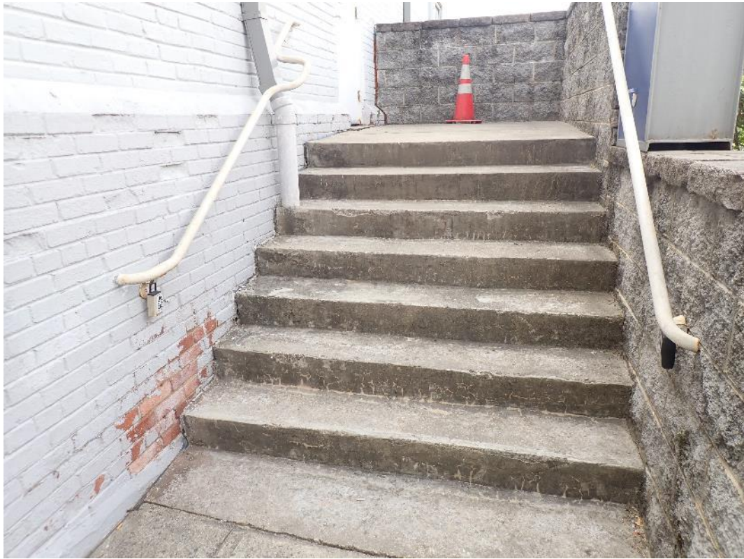
Photograph 11: Exterior steps to the south of the main entrance which have structural issues
