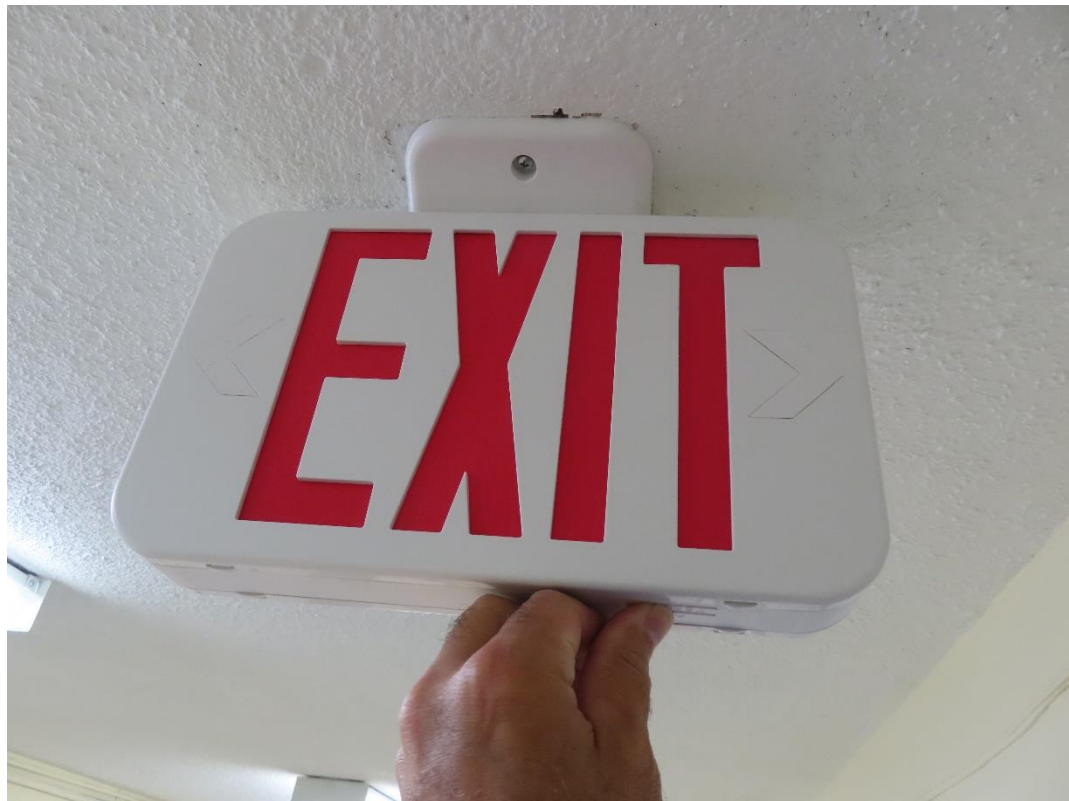
Photograph 47: Non-operational battery backup to internal egress light.
