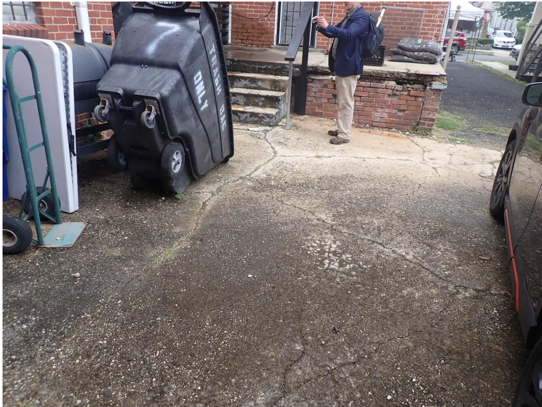
Photograph 9: Cracked concrete paving.
