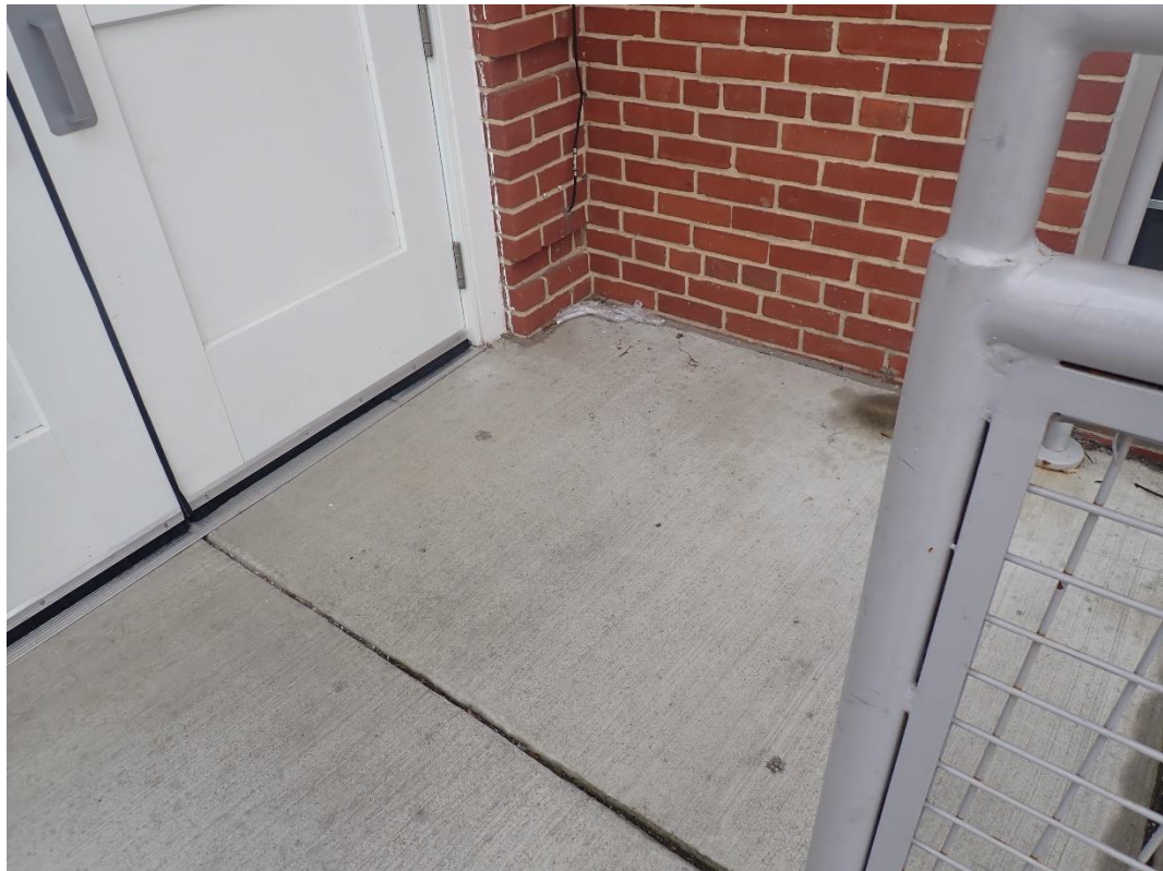
Photograph 2: Inadequate space provided at the top of the accessible ramp
