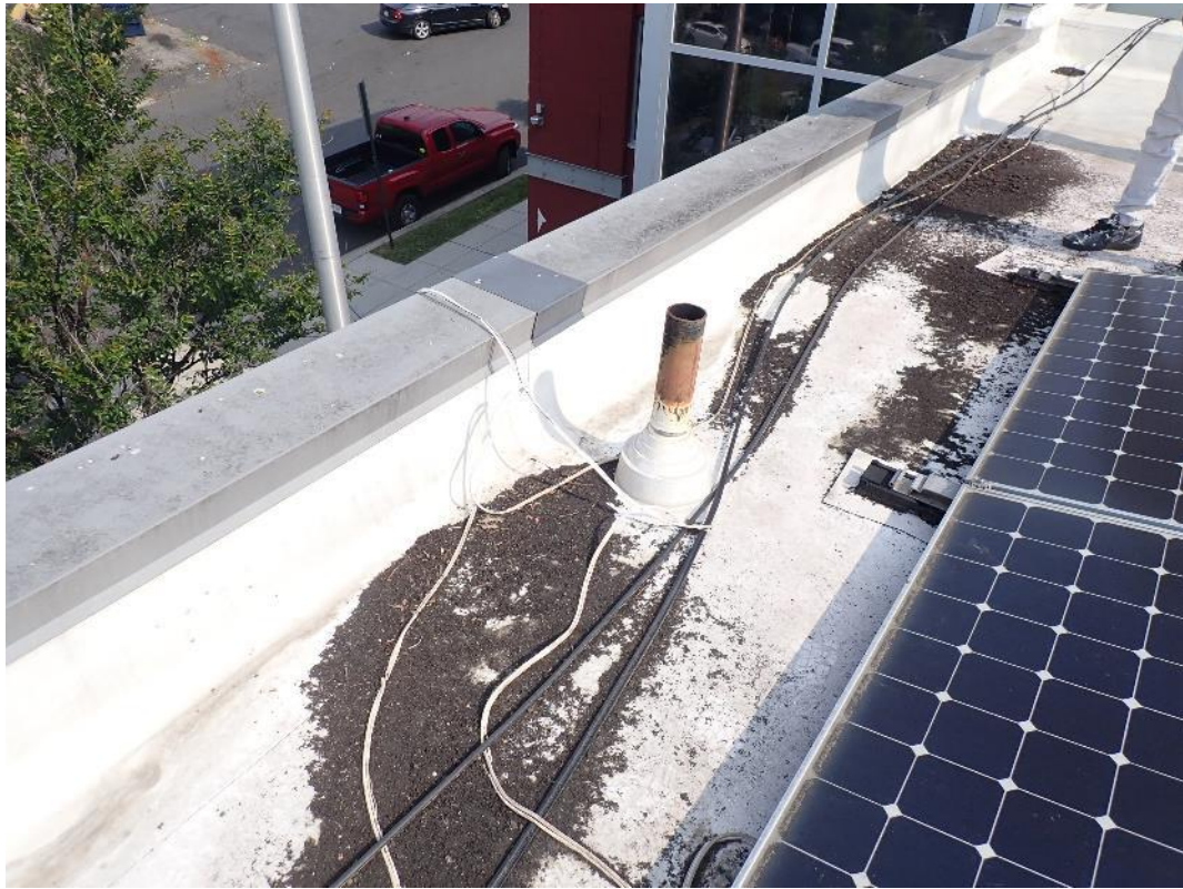
Photograph 19: Debris accumulation on roof.
