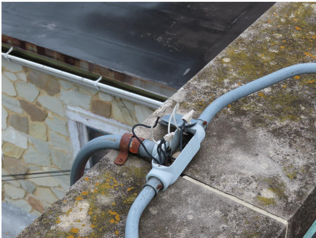
Photograph 40: Exposed electrical connections.
