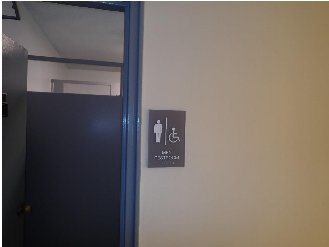
Photograph 4: Accessible signage to non-accessible restrooms.
