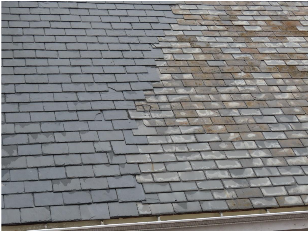
Photograph 13: Misalignment of slate materials and slipped and damaged slates.
