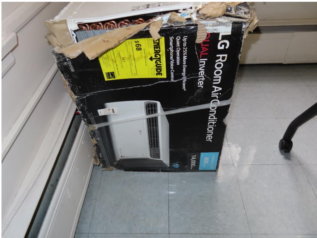
Photograph 28: Baseboard radiators and spare window A/C unit.
