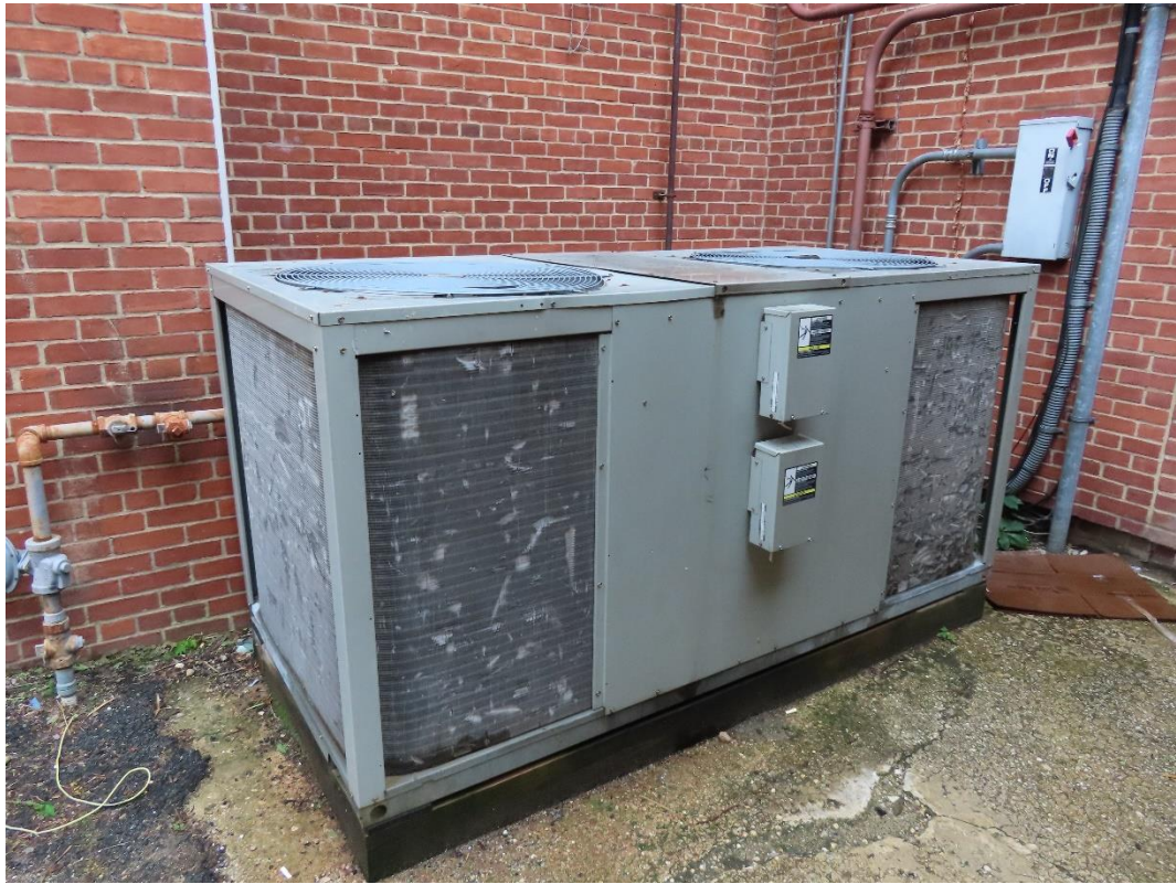
Photograph 23: 20 ton exterior condensing unit
