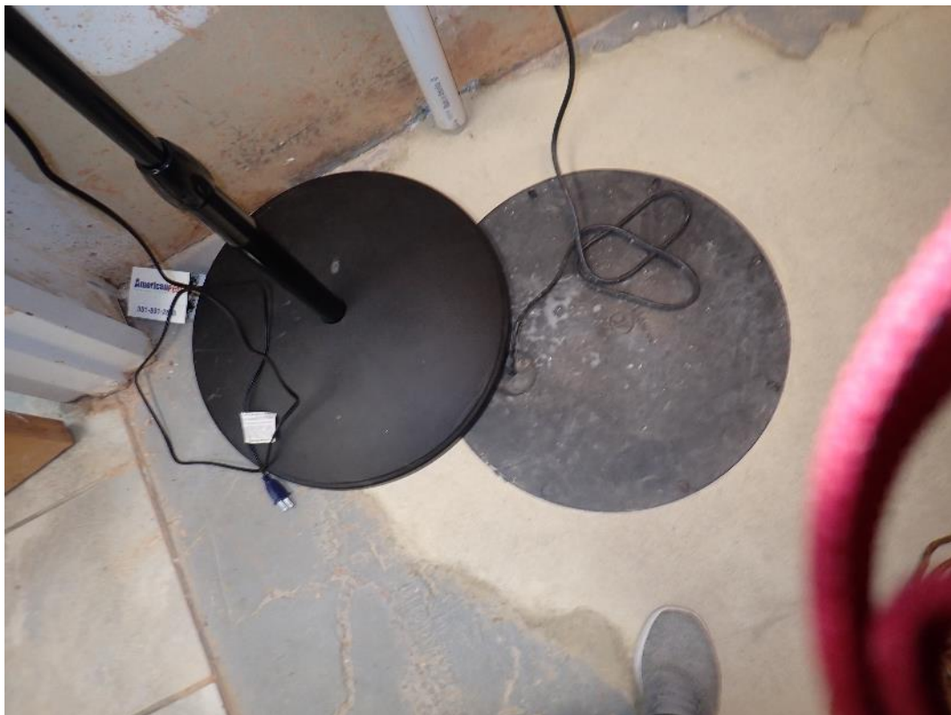
Photograph 40: Sump pump in basement area.
