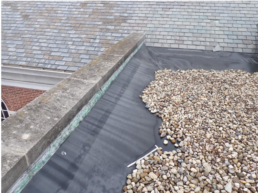
Photograph 12: "Tenting" of ballasted EPDM roofing.
