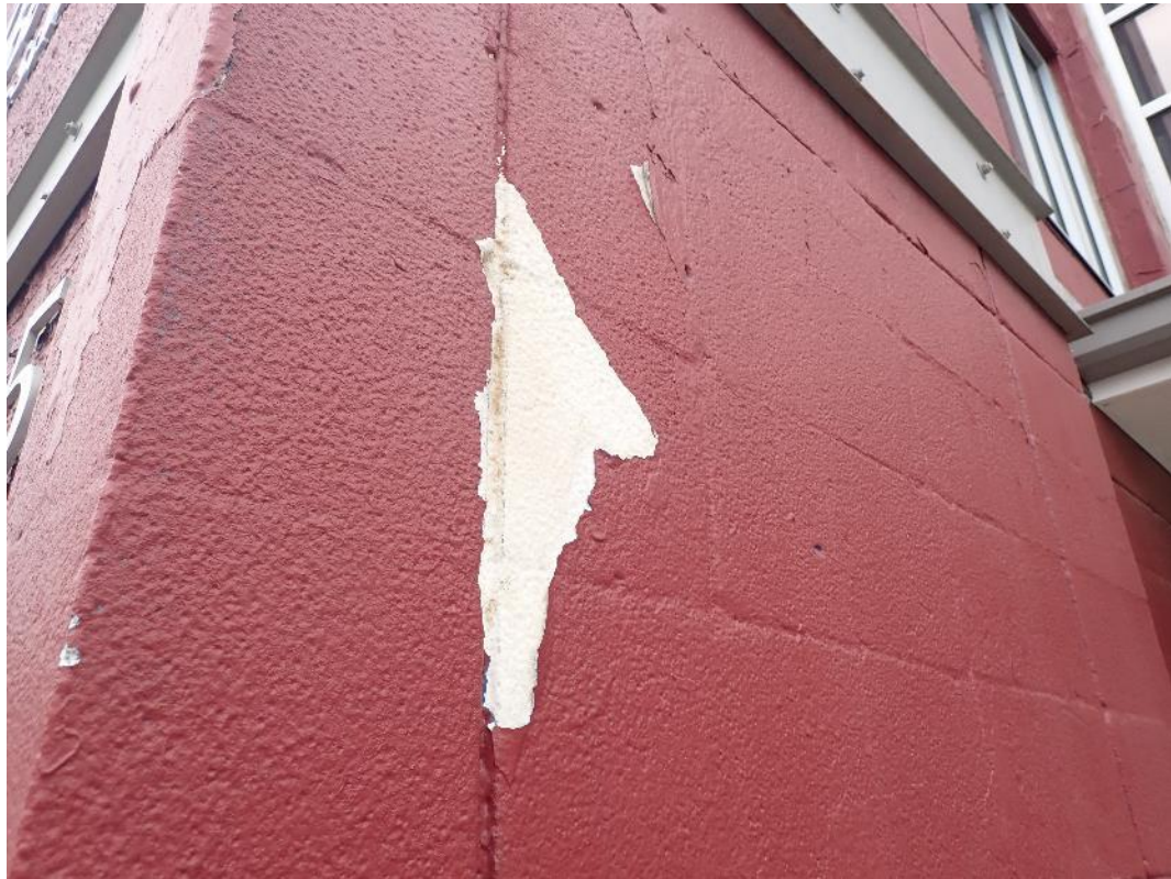
Photograph 23: Deteriorated paint finishes at main entrance area.
