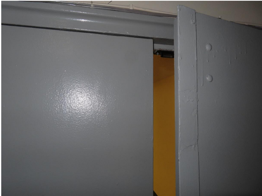
Photograph 49: Flange restricting operation of egress doors
