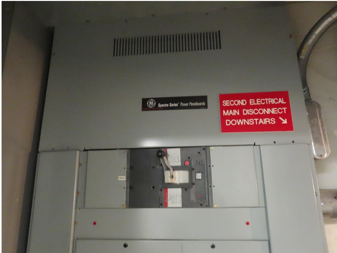
Photograph 41: GE main disconnect.
