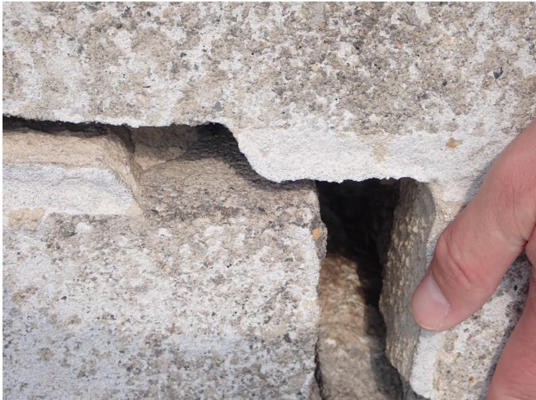
Photograph 14: Extensive structural cracking at exterior wall.
