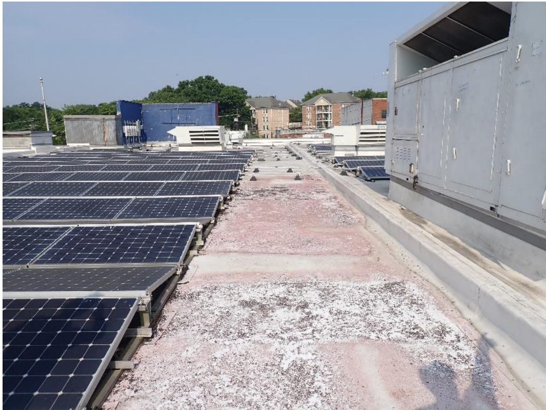
Photograph 17: Staining and debris on TPO roof from excessive water/drainage issues.
