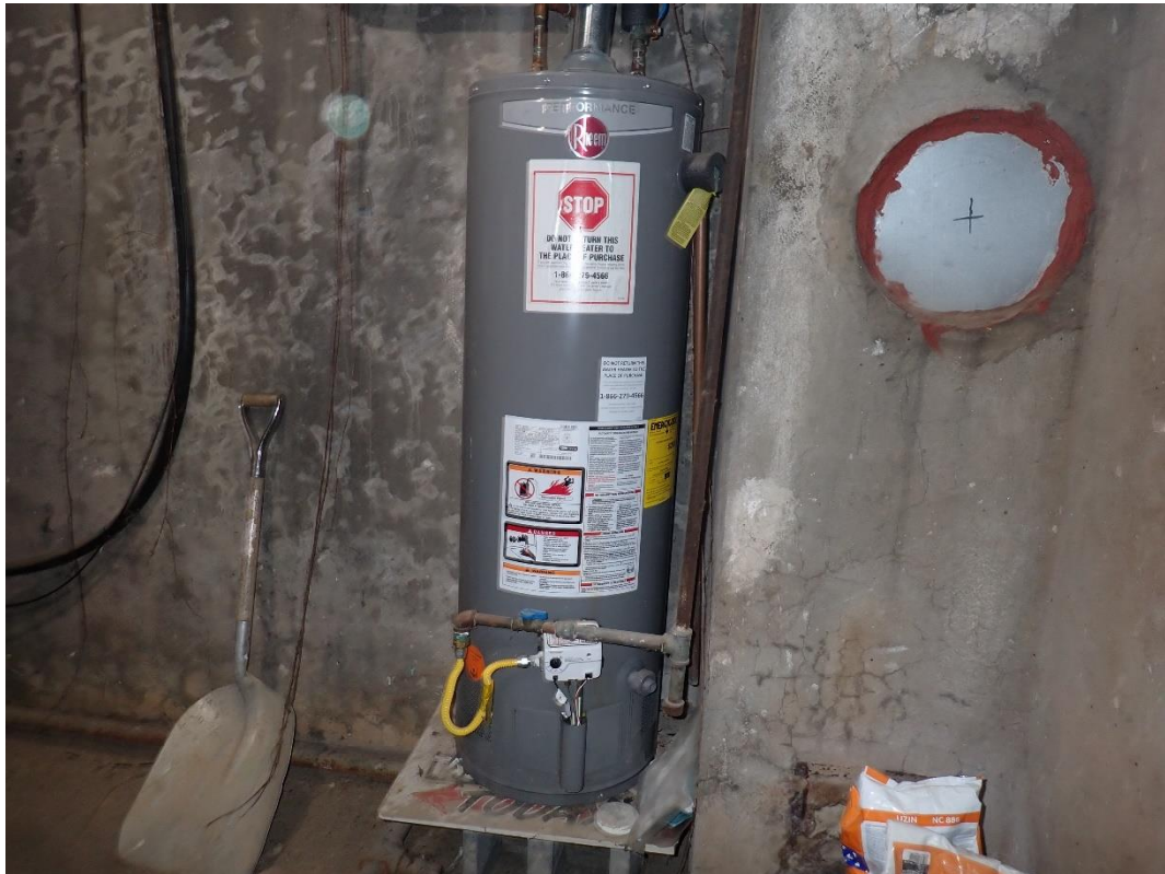
Photograph 45: Hot water heater.
