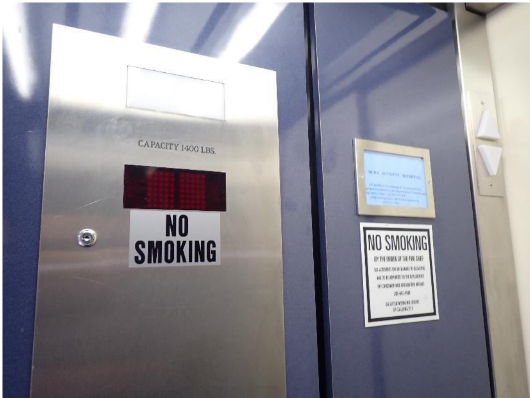
Photograph 47: Elevator car control panel and cab finishes.
