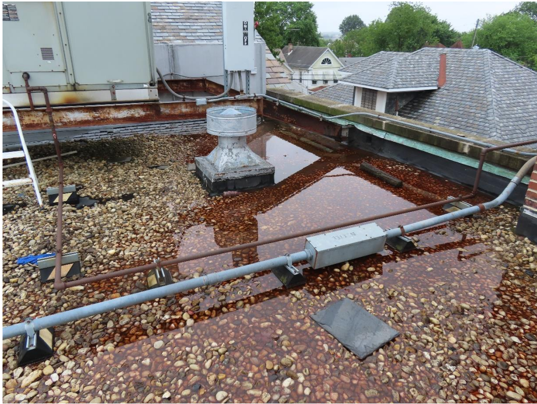
Photograph 11: Ponding water at roof level
