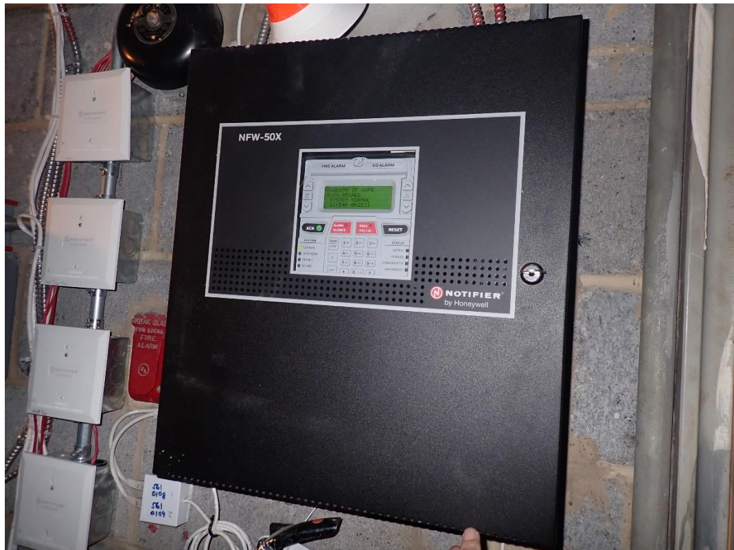
Photograph 51: Fire alarm panel.
