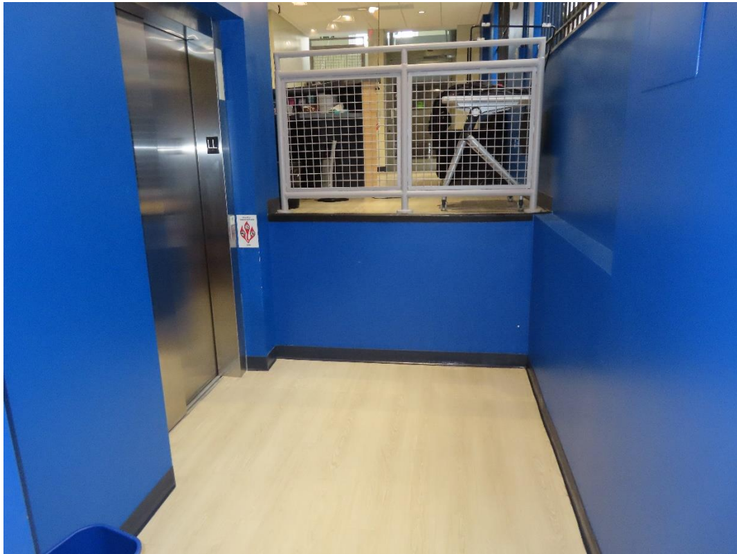
Photograph 53: Machine room-less elevator entry at lower ground floor.
