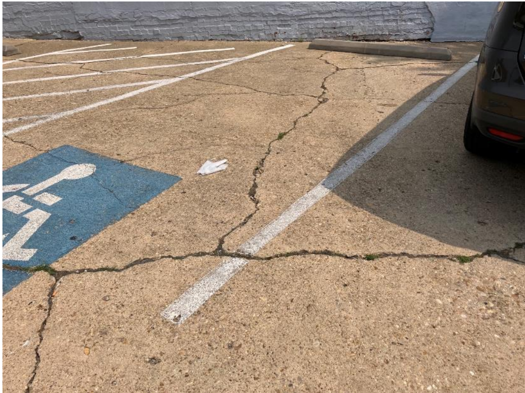
Photograph 7: Cracking to concrete paving at parking area.
