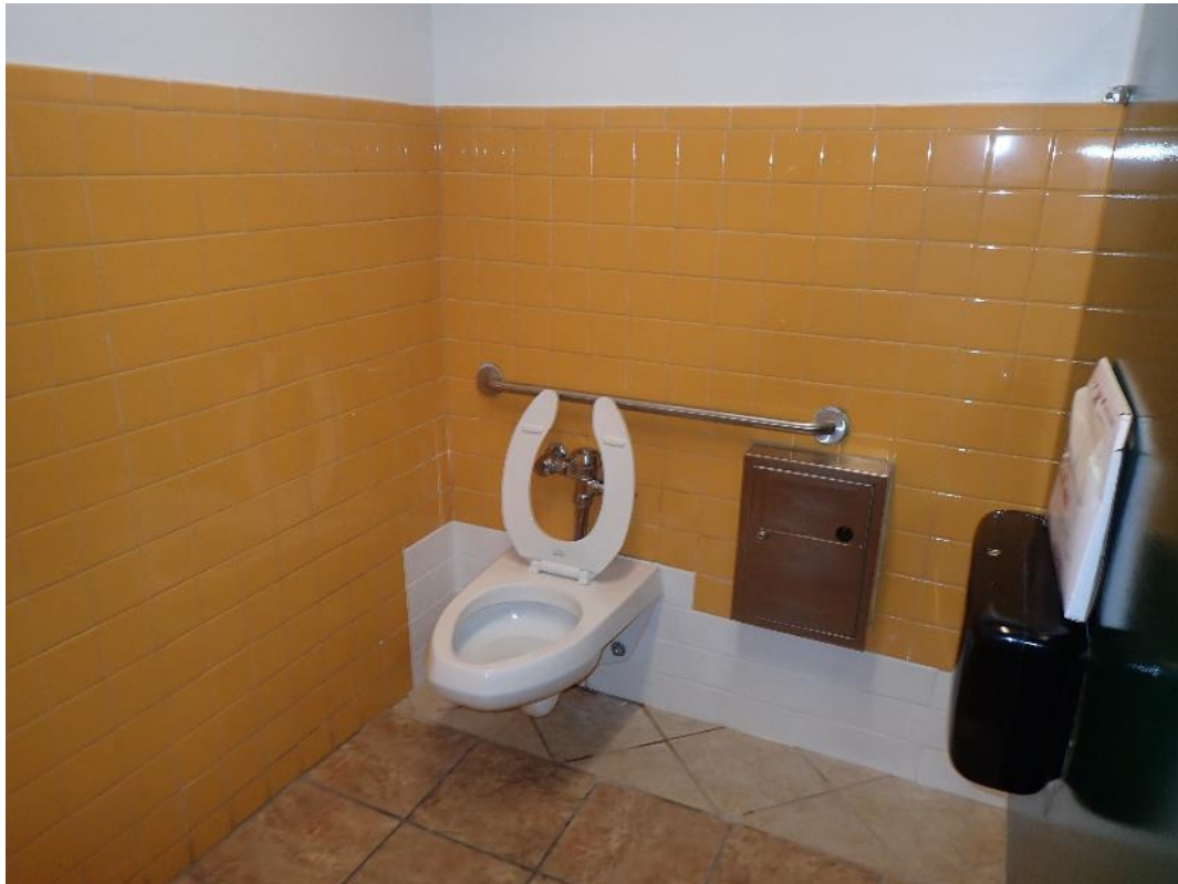
Photograph 3: Accessible stall (note: missing handrail to left-hand side).
