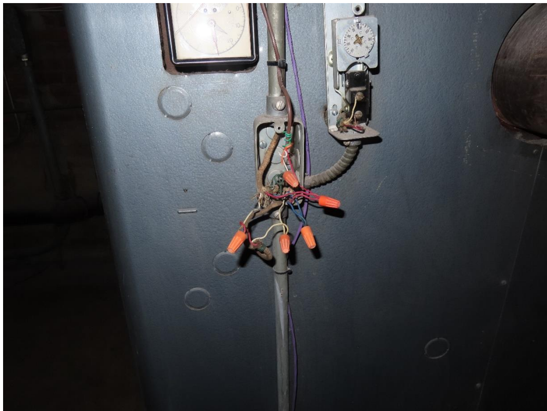
Photograph 38: Exposed electrical connections.
